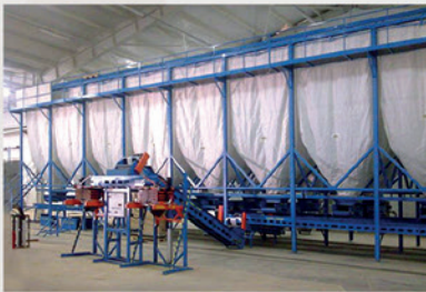
EMVE Storage and feeding hoppers
