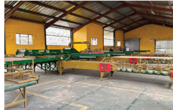
The new potato washing and sorting facility at the Mthatha fresh produce market.
