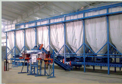
EMVE SWEDEN Storage and feeding hoppers
